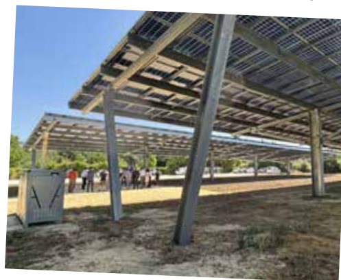
Ombrières de parking, Sainte-Soline
